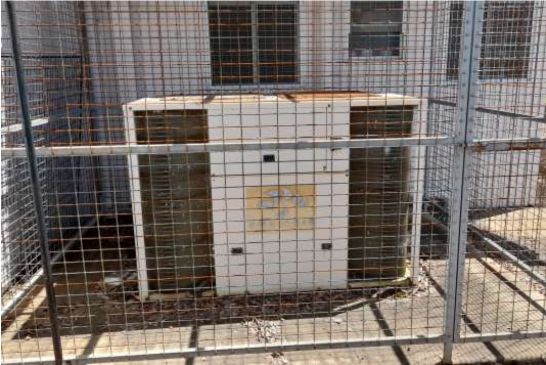
Figure 3: Existing central air-conditioning system (outdoor unit)
