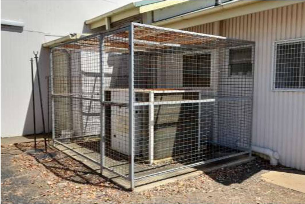
Figure 2: Existing central air-conditioning system (outdoor unit)
