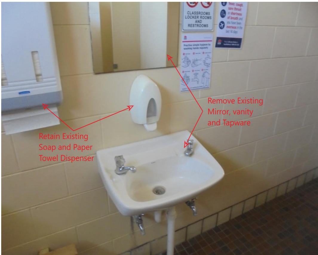
Figure 12. Demolish and remove existing vanity basin, mirror and tapware. Existing soap and Paper towel dispensers to be reinstated
