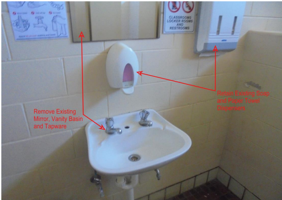
Figure 6. Demolish and remove existing vanity basin, mirror and tapware. Existing soap and paper towel dispensers to be reinstated
