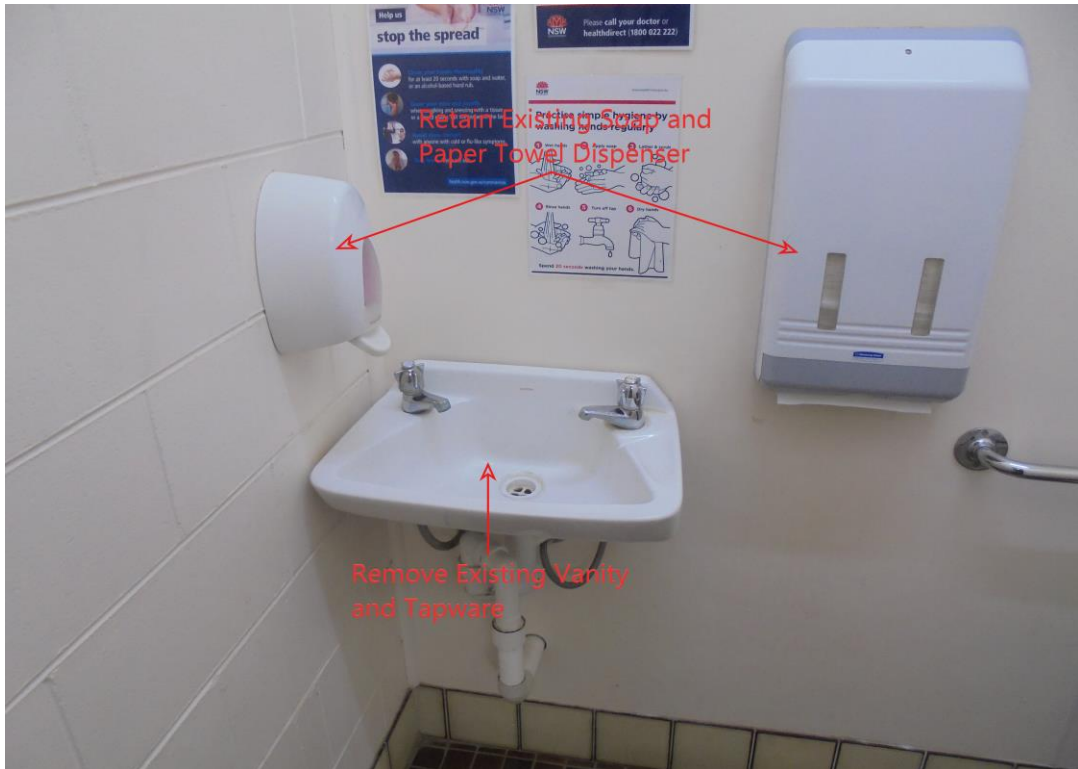
Figure 18. Demolish and remove existing vanity basin and tapware. Existing soap and Paper towel dispensers to be reinstated
